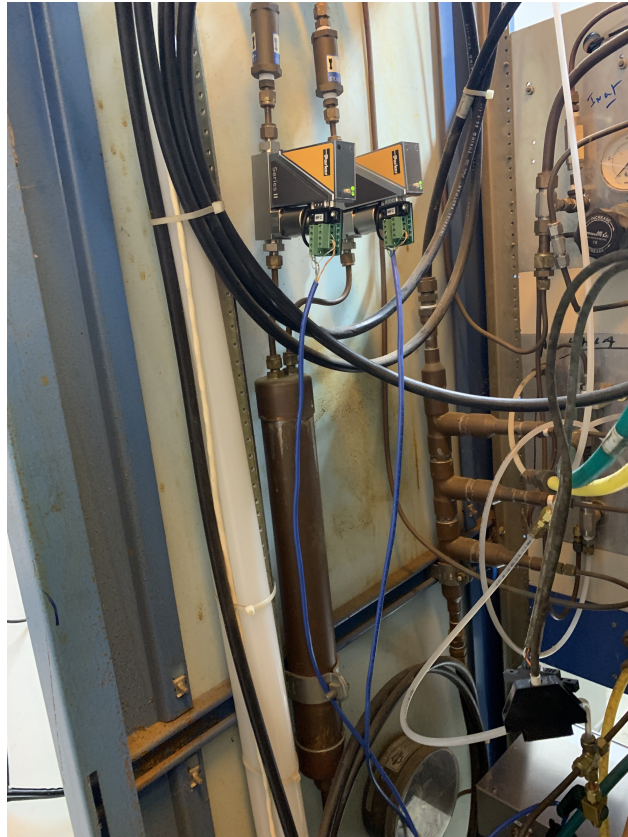
Figure 21: MFCs (orange, black, and green) are near the top and the metal cylinder is the mixing tank (below MFCs near middle of picture) for BigBite GEM.
