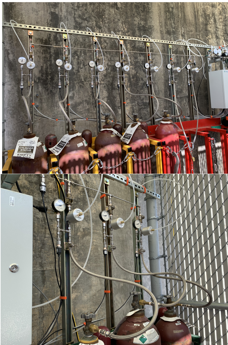
Figure 27: SBS GEM regulators and cylinders
