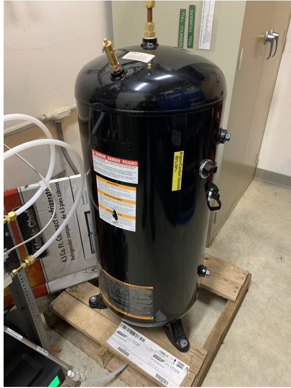
Figure 30: SBS GEM Buffer Tank
