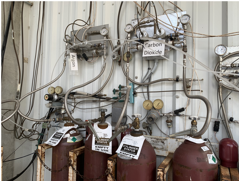
Figure 20: BigBite GEM regulators and cylinders.
