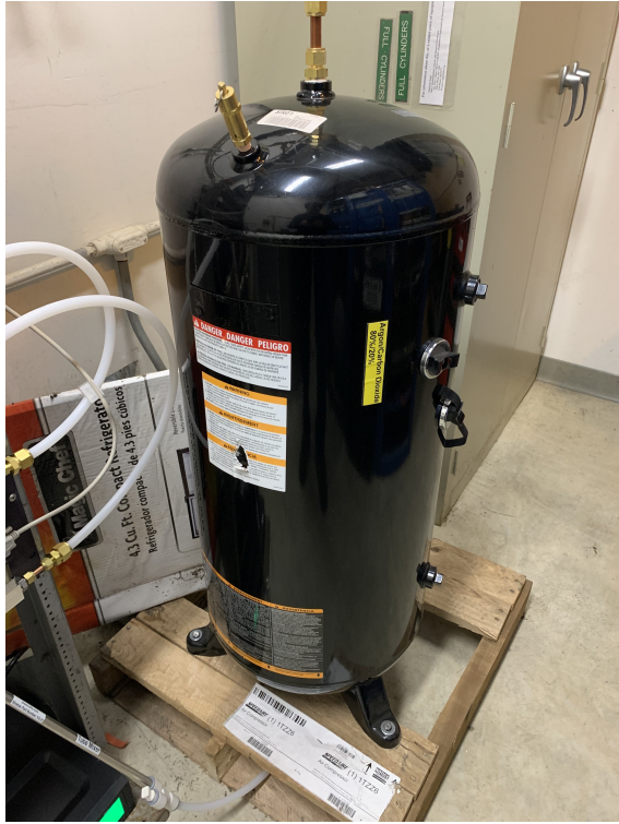
Figure 31: SBS GEM Buffer Tank
