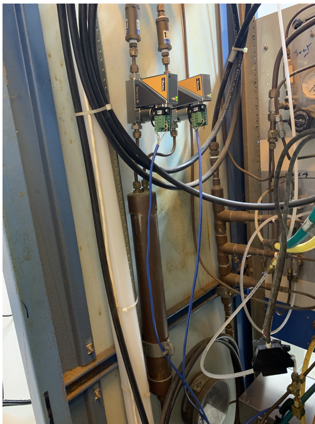
Figure 22: MFCs (orange, black, and green) are near the top and the metal cylinder is the mixing tank (below MFCs near middle of picture) for BigBite GEM.
