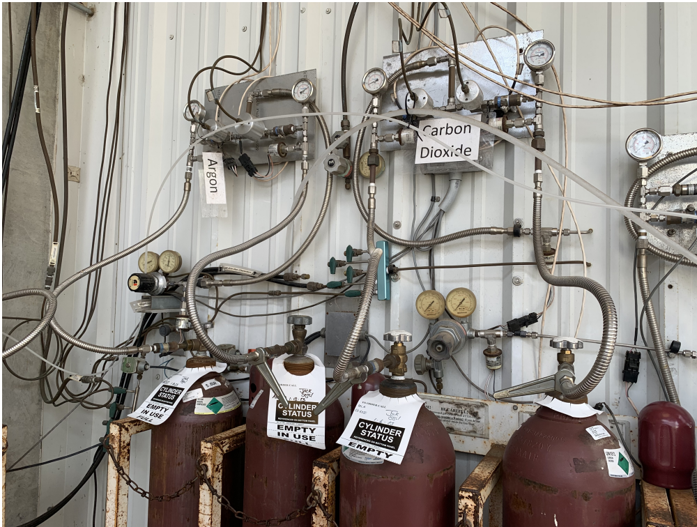
Figure 21: BigBite GEM regulators and cylinders.
