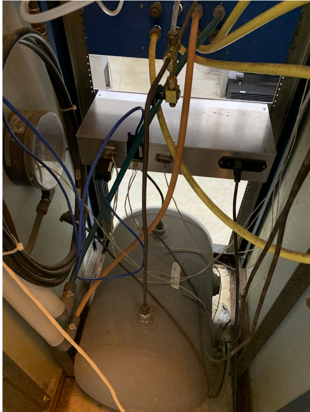
Figure 26: BigBite GEM buffer tank and purge valve.
