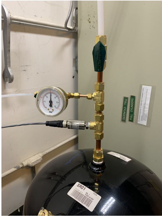
Figure 34: SBS GEM Gas Shut Off Valve, in this picture valve is open
