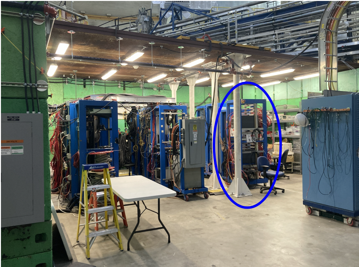
Figure 4.2: HCAL-J HV Crates Located in the DAQ Bunker.
